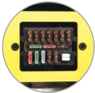
Concentrated Fuse Box for Easy Inspection
